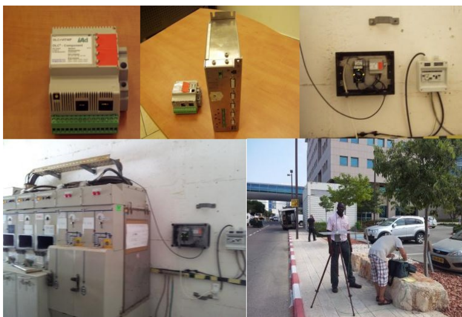
Figure 1: Modem Installations; Performance and EMC Measurements
